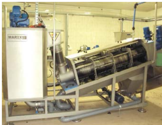
A modern press for sewage treatment plant in Lisków worth PLN 541,200 was purchased for funds obtained under the RDP for 2014-2020.
